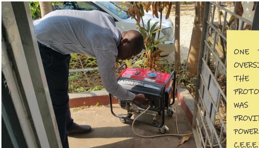
Figure 52: Starting the generator during a blackout at the CEEEZ office.
