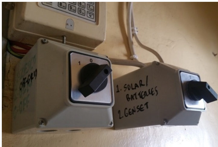
Figure 59: The final installation allowed CEEEZ to switch almost seamlessly between solar, generator & ZESCO grid power supplies. The batteries could charge from solar during the day and on cloudy days with high energy demand, they could be topped up from the grid.
