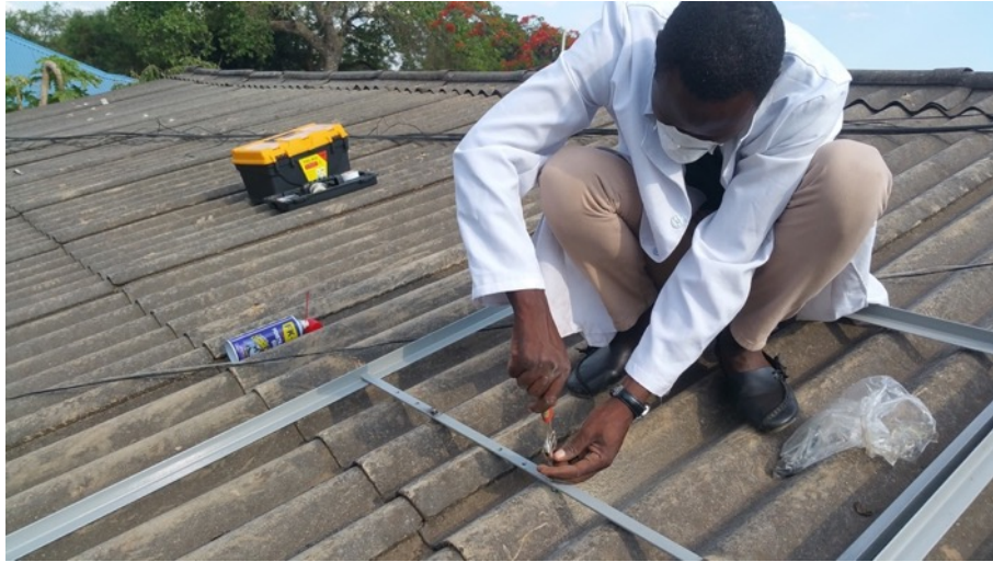
Figure 53: Installing the mounting frame for the PV on the roof of the CEEEZ office.
