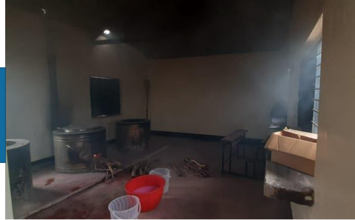
Case 5: Primary school in Kakuma, three 100L stoves to cook for 2400 children. Smoke fills the kitchen (picture 2) when the stoves are lit due to broken chimneys.
