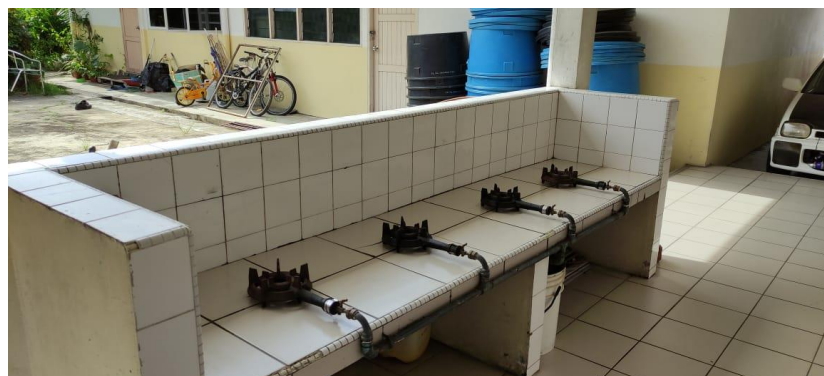
Figure 4.6 Stove with Gas pipeline in Red Cross Miri Branch
