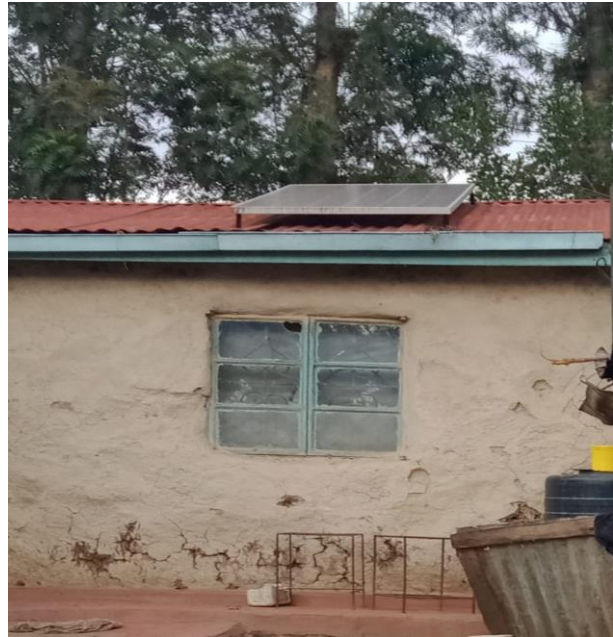
Figure 8: Picture of solar panel installed above the roof of Gibson's home. (Photo credit: Emily, ACTS)
