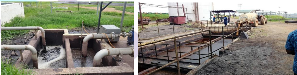
Figure 3.5 Effluent from the mill being disposed and channelled into the biogas reactor
