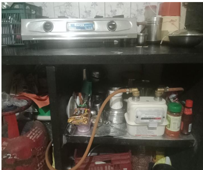
Figure 3: Gas meter installation at a lower income household
