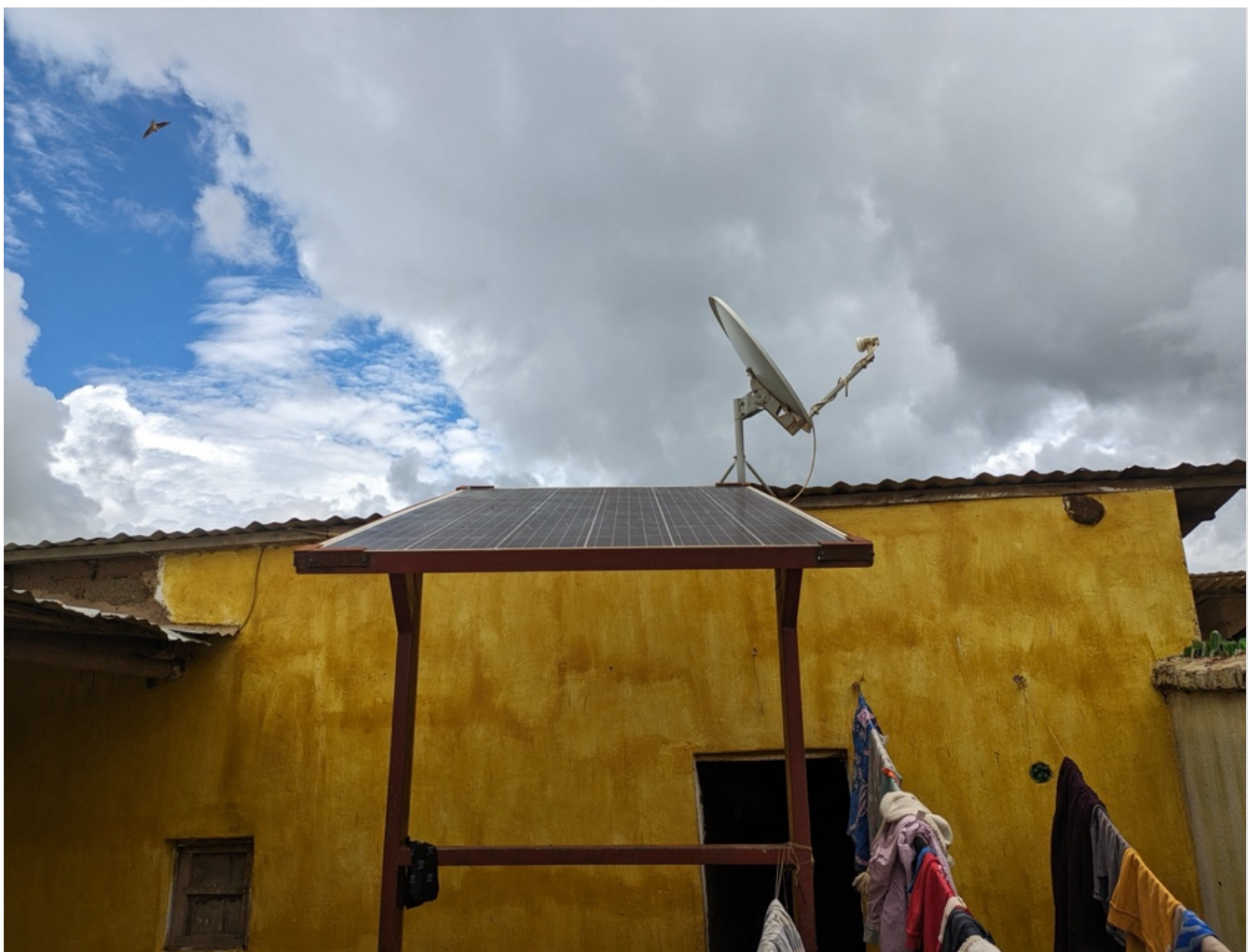
Image 14: A solar panel installed in a beneficiary compound (JFT, January 2024)
