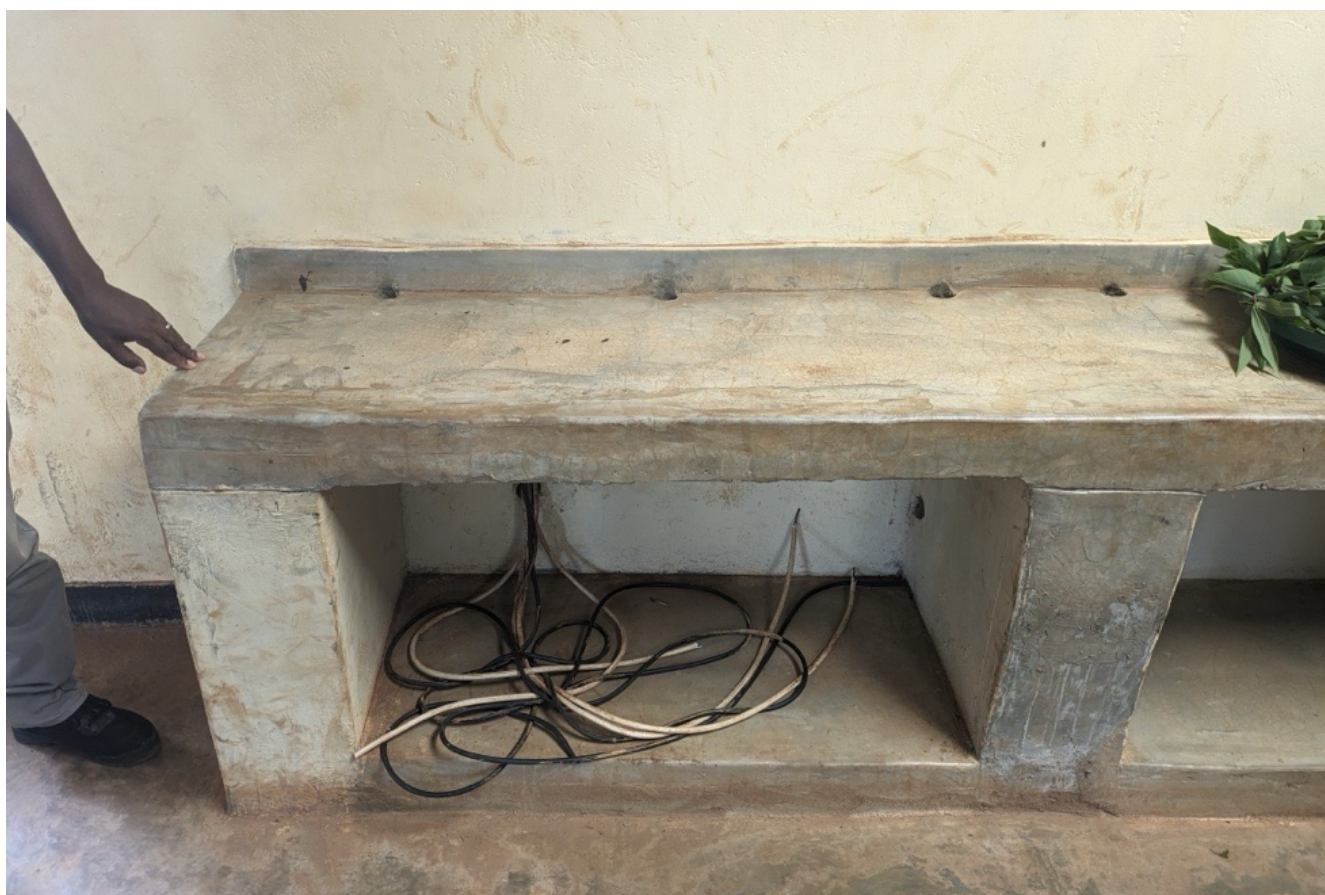
Image 16: Dedicated space for ECOCA with wiring in Day-care Centre (JFT, January 2024)
