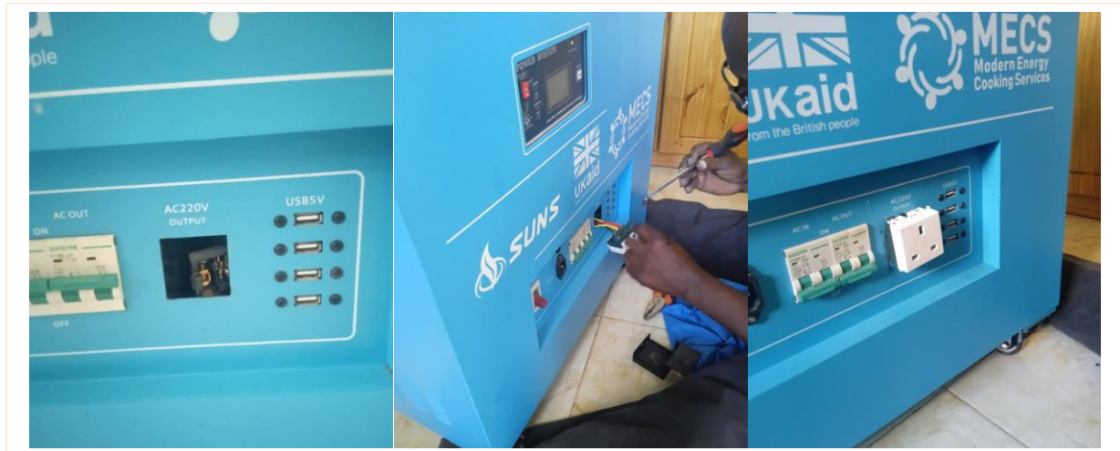
Photos showing the Powerhub which its outlet socket had broken, technician replacing the socket and the hub after replacement.
