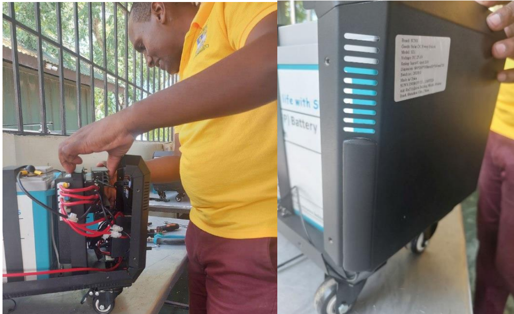
Technician fixing the DAQ to the Powerhubs at TaTEDO-SESO clean cooking centre.
