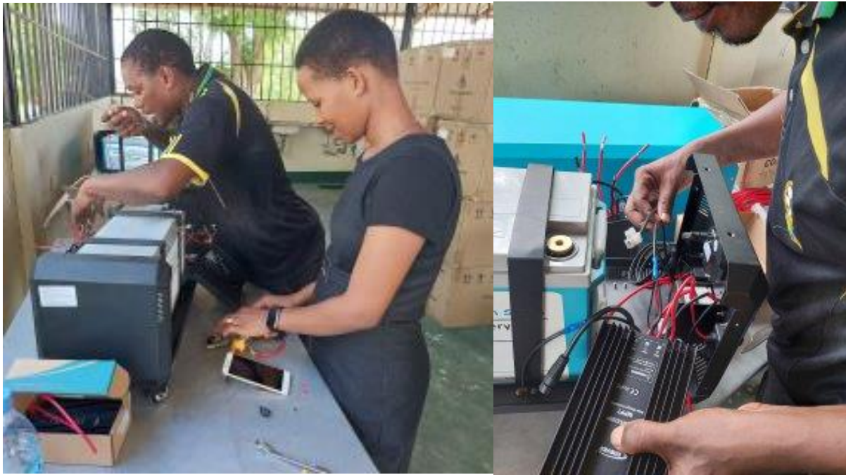
Technicians upgrading the systems at TEDO-SESO Facilities.
