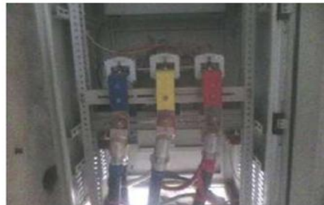
Thermal imaging of supply interface
